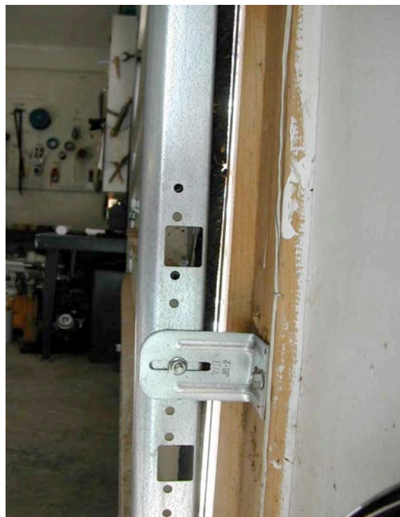
Poorly-fitting garage door at Parks & Recreation.
