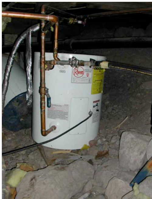
Town Hall's water heater in a cold, un-insulated crawlspace, with bare copper pipes. Heat loss anyone?
