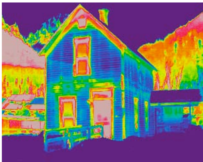
Infrared image of Nordic Center showing heat loss at windows and house corners and attic vent.
